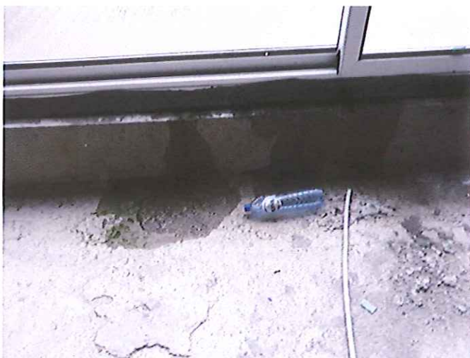
infiltration Appart 3 eme
